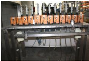
Reference: BPS-066 PUMP GROUP Year: . Brand: PROMINENT
