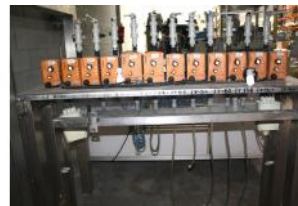
Reference: BPS-066 PUMP GROUP Year: . Brand: PROMINENT
