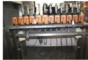
Reference: BPS-066 PUMP GROUP Year: . Brand: PROMINENT
