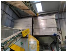
Reference: MZA-007 STORAGE HOPPER Year: 2018 Brand: .
