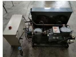
Reference: MOR-241 COOLING UNIT Year: 2001 Brand: .
