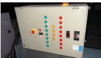
Reference: MOR-244 COOLING UNIT Year: 2001 Brand: C+F
