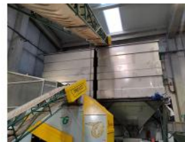
Reference: MZA-008 STORAGE HOPPER Year: 2018 Brand: .
