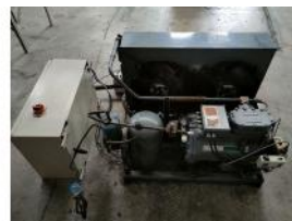
Reference: MOR-241 COOLING UNIT Year: 2001 Brand: .
