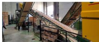
Reference: MZA-005 CONVEYOR BELT Year: 2018 Brand: TREICO
