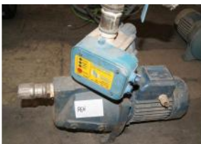
Reference: CFG-017A PUMP CENTRIFUGAL Year: . Brand: .
