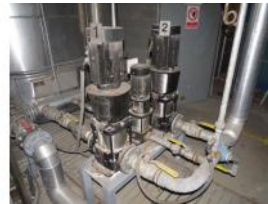
Reference: SER-084 PUMPS Year: . Brand: .
