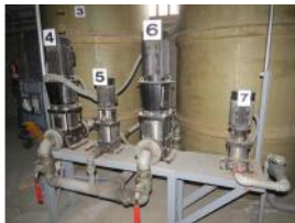
Reference: SER-083 PUMPS Year: . Brand: .
